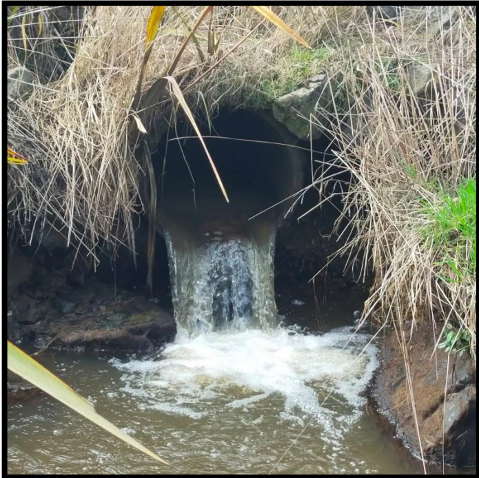
Image 2 – Perched culvert on downstream side of unnamed tributary at Middleton Road. Date taken: 10 / 09 / 2023. Source: Jacob Smyth.
