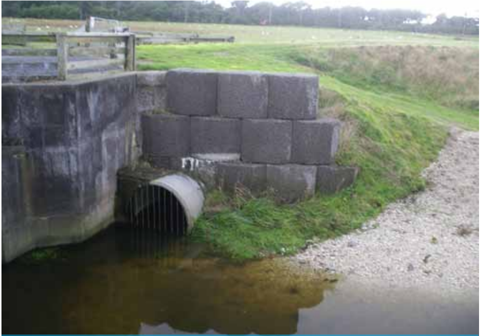
A reticulated stormwater drain.
