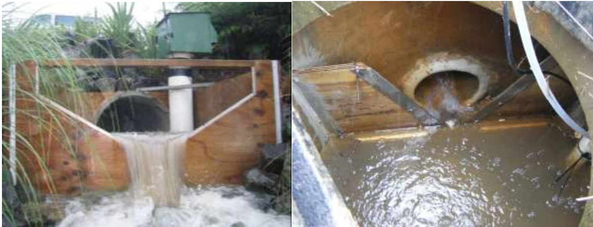
Figure 5-1: Examples of temporary sharp-crested weirs constructed for stormwater monitoring of an outfall pipe (using a weir box) and within a manhole.
