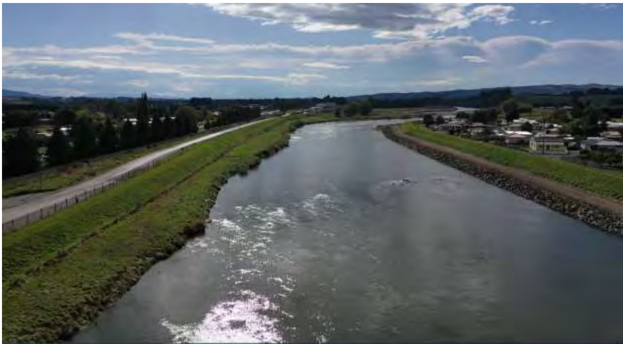
Mataura true left bank berm rock lined and true right bank berm not rock lined
