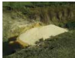
▶ A large pile of soil can provide a temporary measure to prevent effluent spreading in a waterway.
