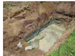
▶ A pit will collect spilled effluent.
