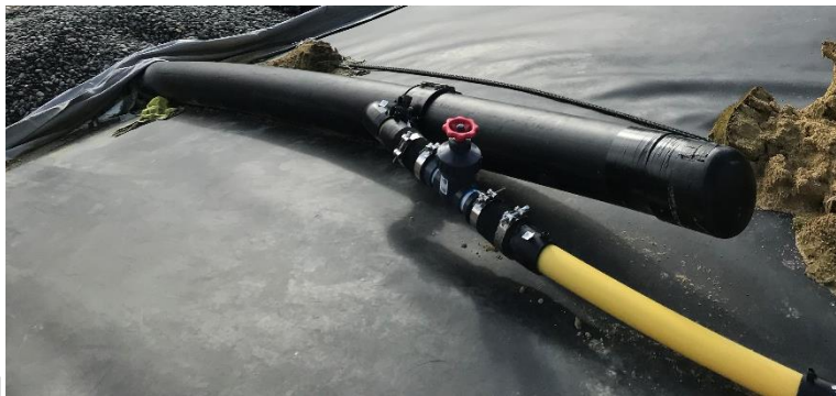
Figure 21 Leachate clean-out pipes extended up the eastern side wall of the landfill (dated 01 August 2019).
