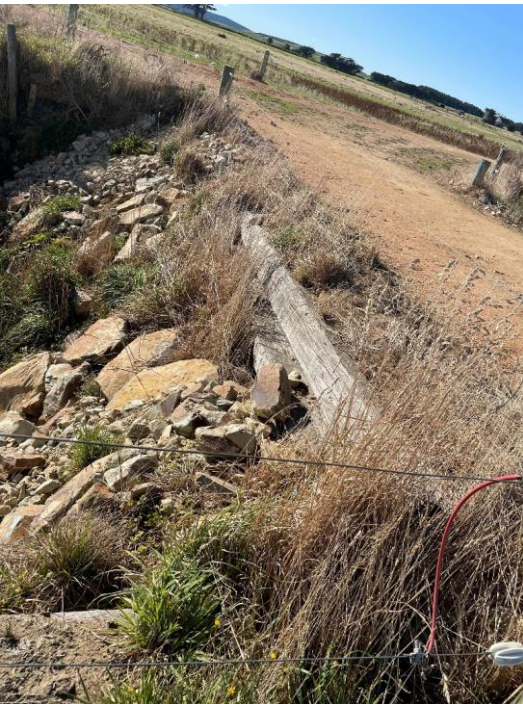
Culvert stock crossing showing vegetative lip (more work is planned on some of these)
