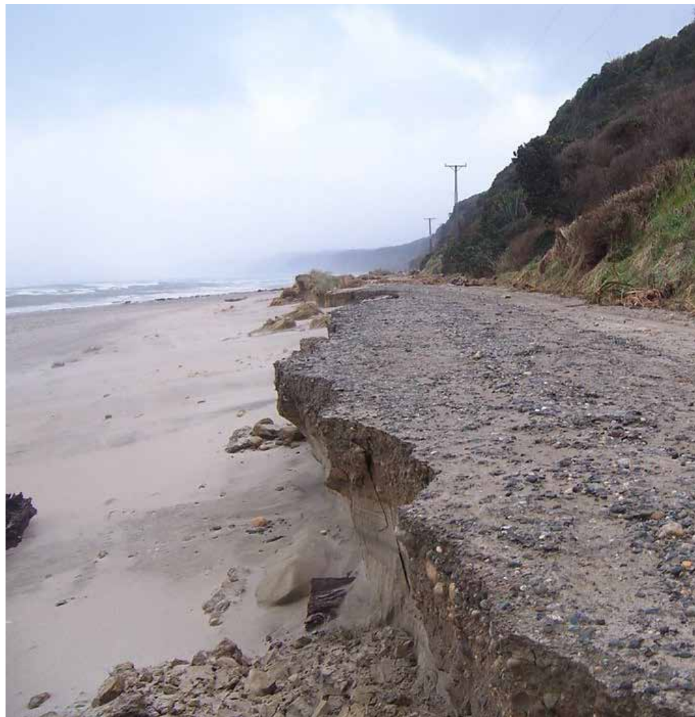
▲ Coastal erosion of the Papatotara Coast Road along Te Waewae Bay (2007)
