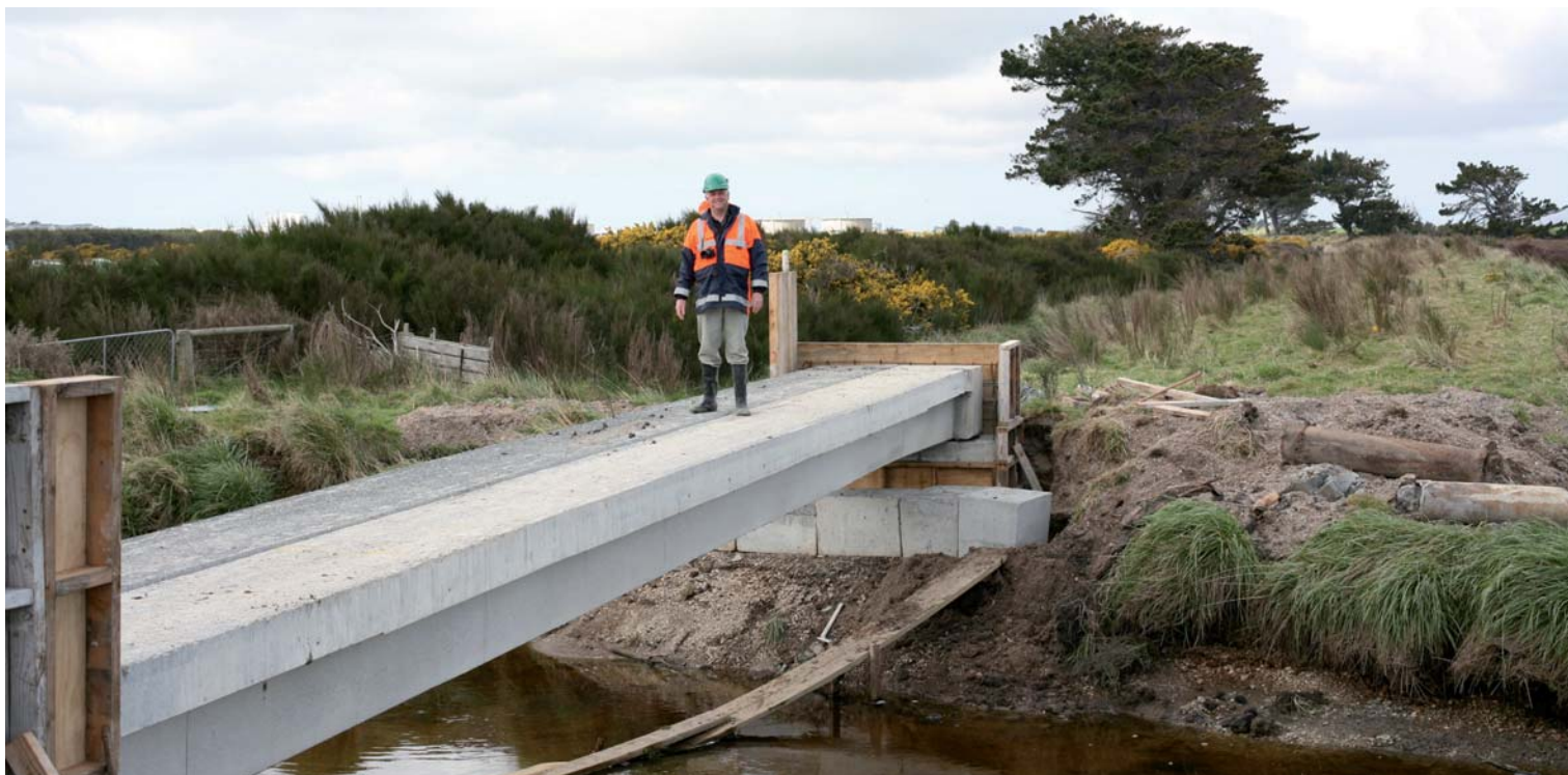
Project manager Robin Wilson, from Environment Southland, on the recycled concrete beams which form the basis of the new walking and cycling bridge across the Kingswell Creek.
