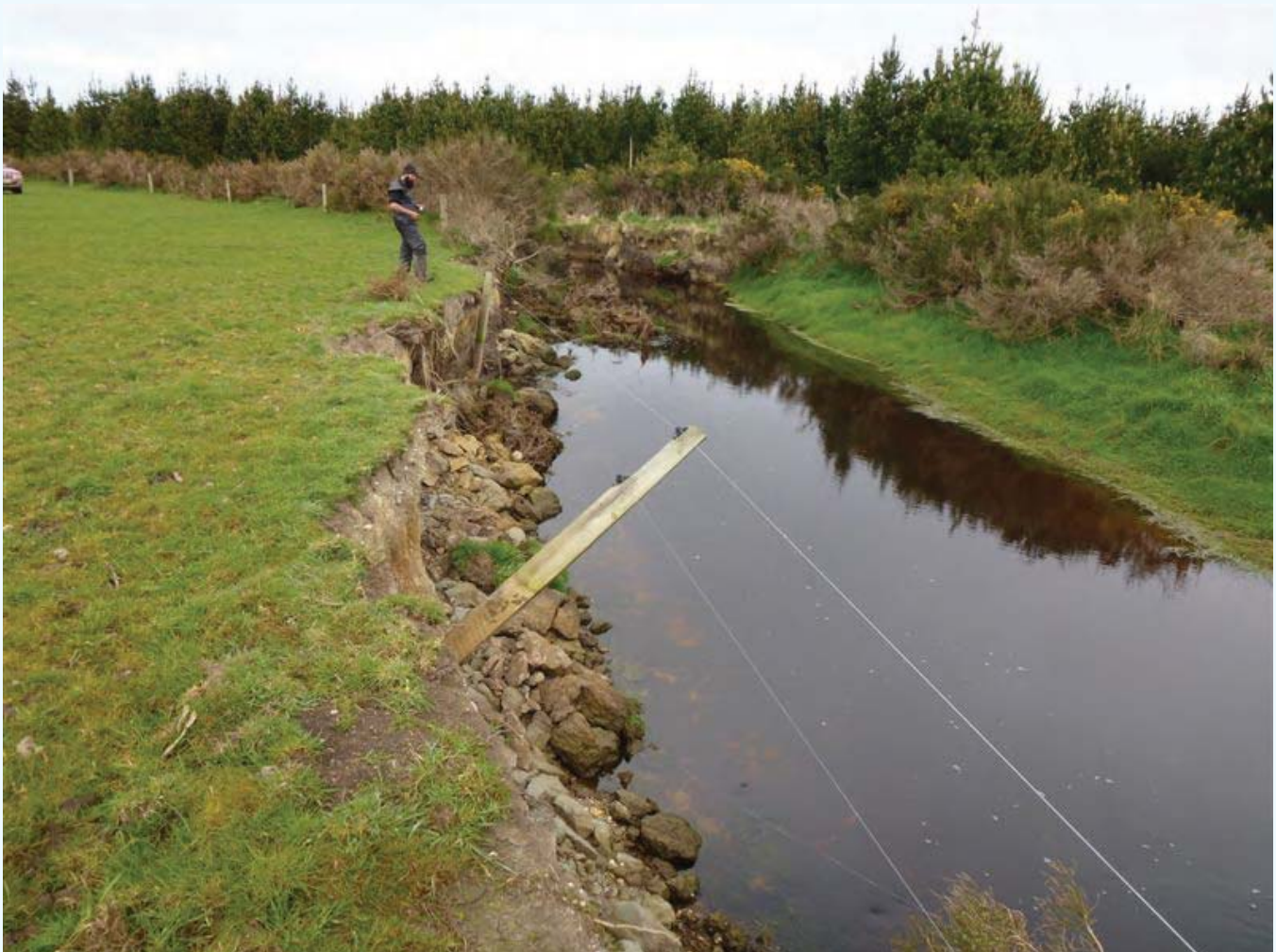
Erosion like this will be the focus of rebattering work on the Waituna Stream.
