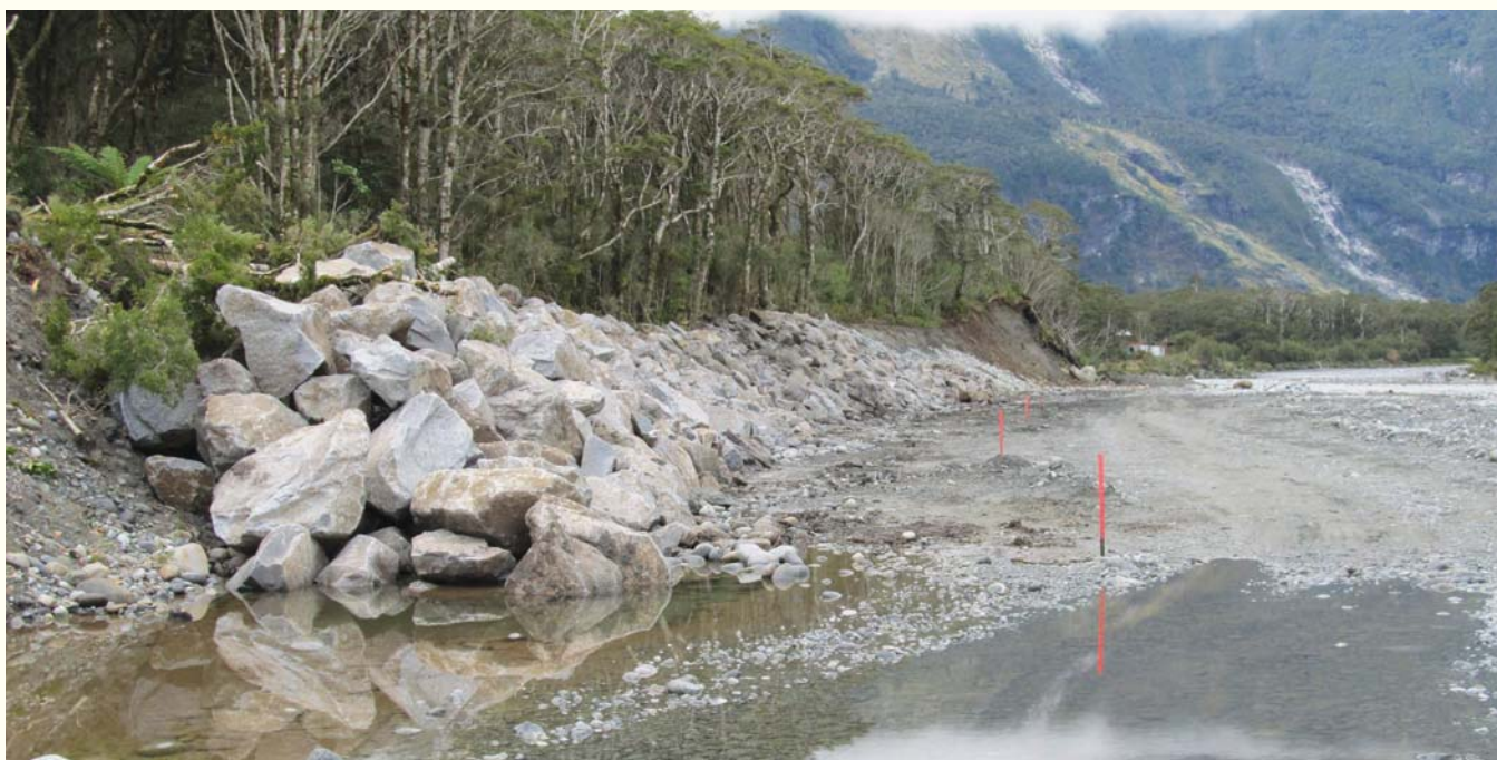
Rock protection has been placed along the banks of the Cleddau River to stop erosion which was threatening the village and the Milford Road. Photo: Noel Hinton.
