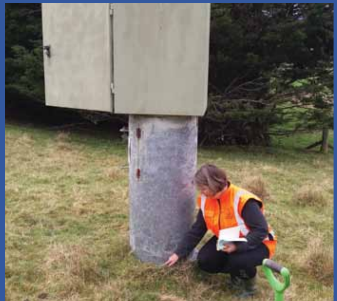
▲ Business systems analyst Lianne Kooiman points out a sea level benchmark on a tower for the Otepuni Stream on a trip with the environmental data team. The tower is used to measure the water level of the stream. It contains pipes which pump water up inside to provide a more accurate environment to measure levels.
