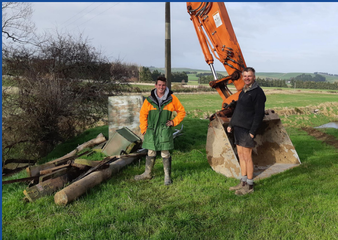
▲ Environmental technical officer Mitchell Harvey and Yorke Excavating Ltd owner Bradley Yorke removing hydrology equipment from the Waikaka Stream at Willowbank. This site has been decommissioned and replaced by a site downstream which can provide improved water flow and water quality data.
