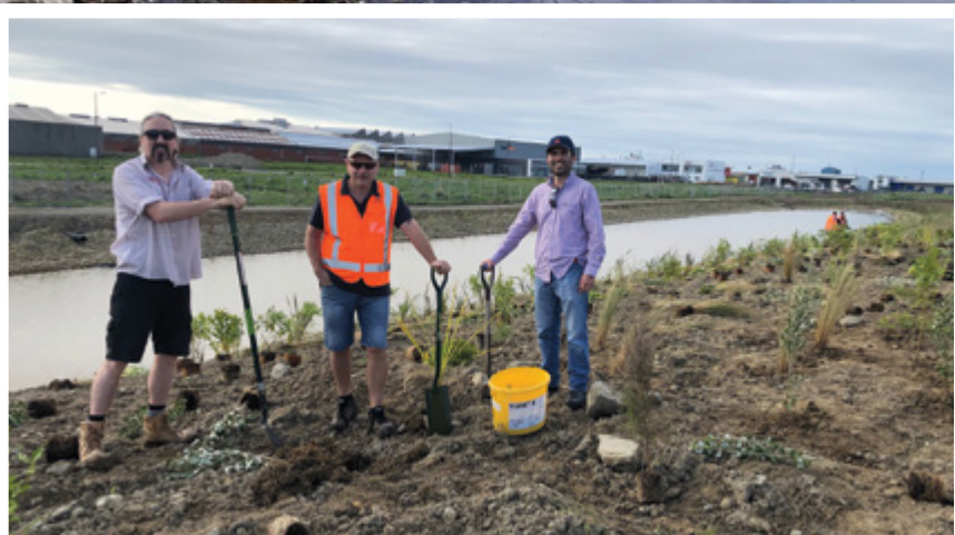
▲ Regan McRandle from The Roading Company, ICC Parks operations manager Chris McAulay and ICC capital projects technician Leonardo Ramirez get busy at a planting day at the new sediment pond.
