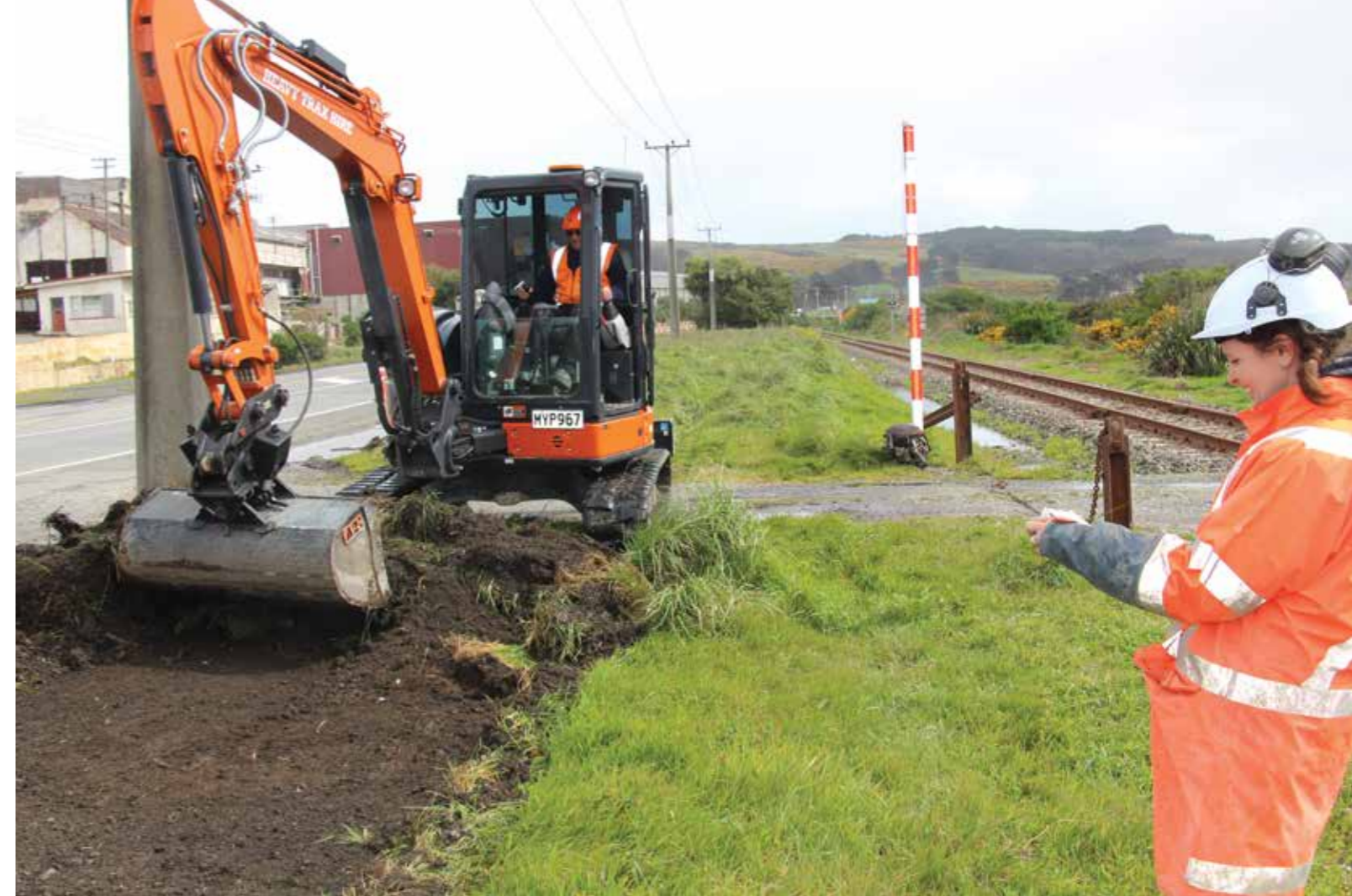
▲ South Roads foreman Mike Bell with Heritage Properties archaeologist Megan Lawrence at the site of the walkway.
