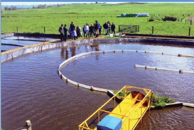
THE HIGH RATE POND (with paddle wheel in foreground and maturation pond cells behind) in the advanced pond system built in Waikato
