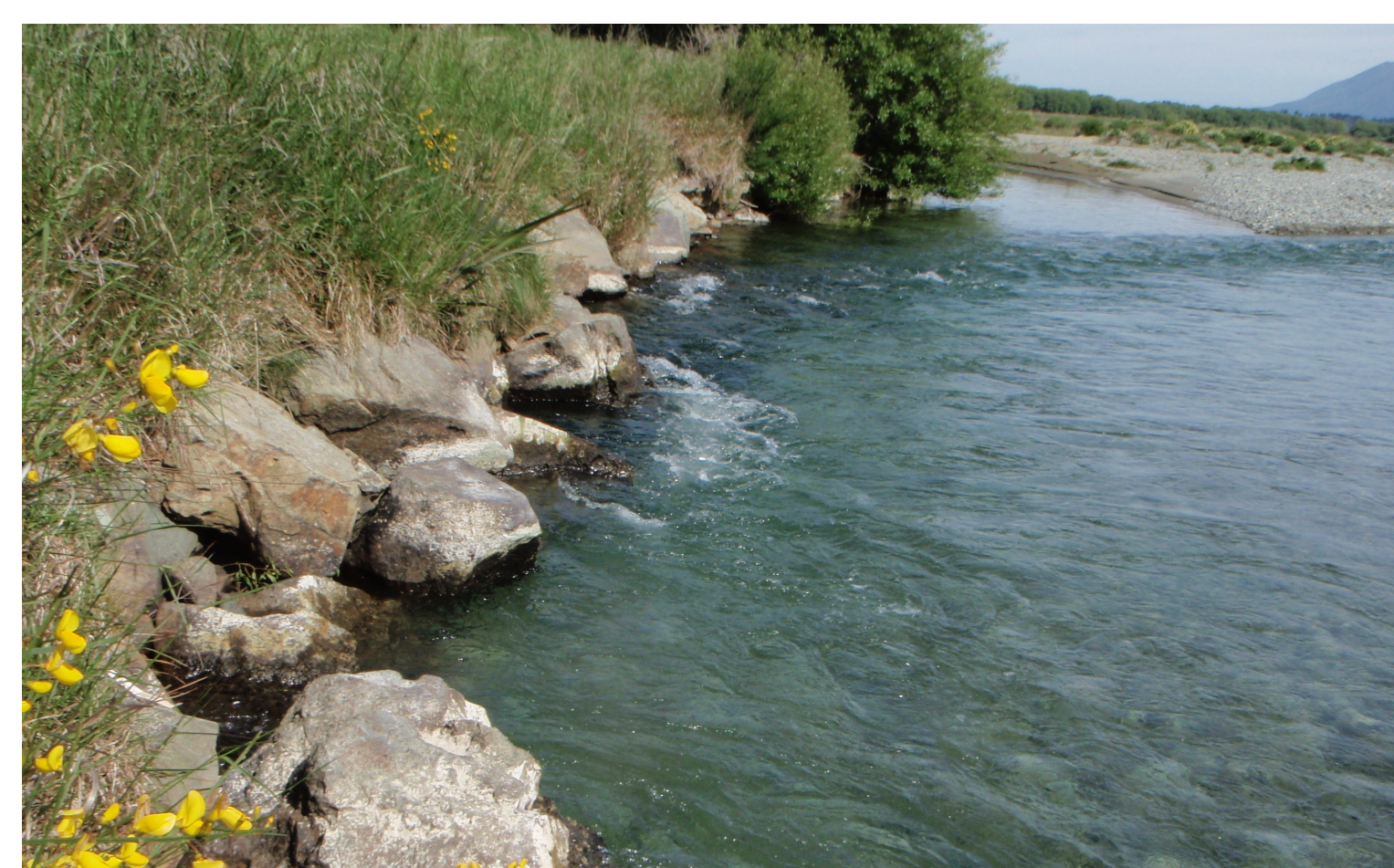
▶ Upper Oreti River – bank erosion arrested by rock protection put in 2007 to protect the bridge abutment.
