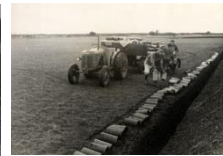
Sub surface drains
