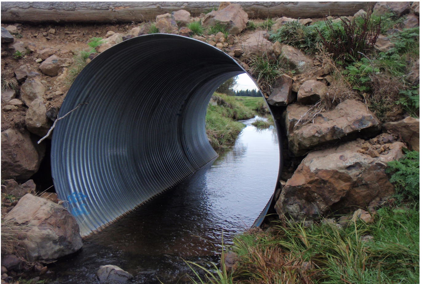
Excellent culvert design providing year round fish access
