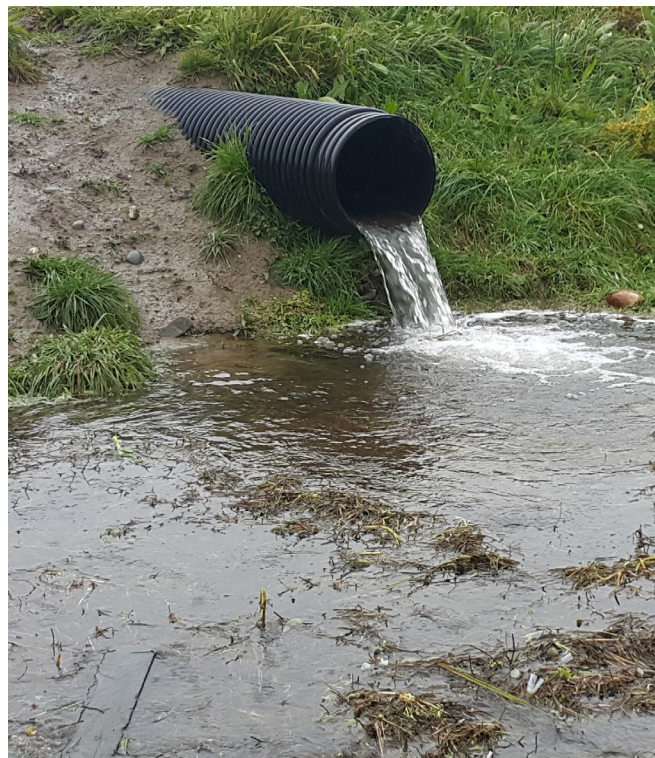
A perched culvert preventing fish access
