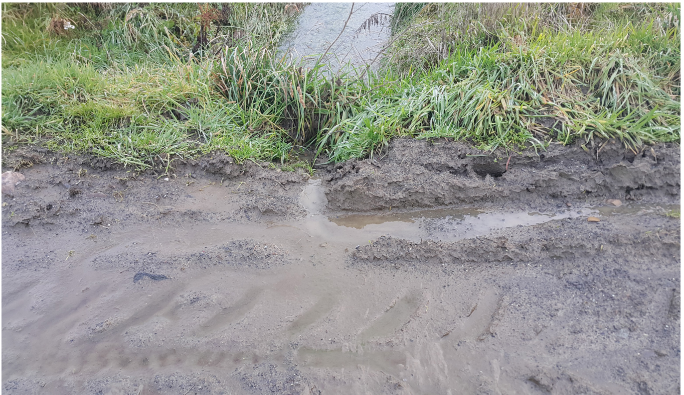
A common leak into a waterway
