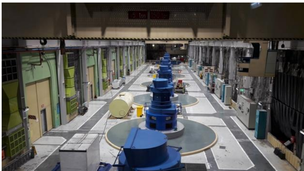
Figure 13: Turbine Hall - Manapouri Power Station
