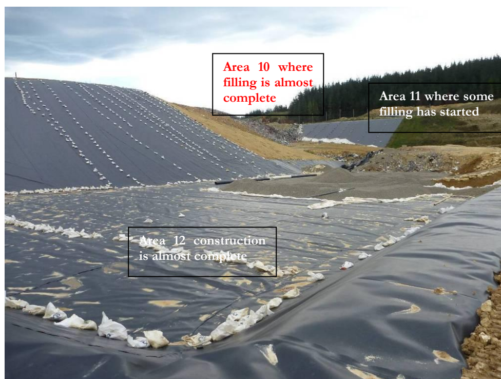
Figure 53: View from edge of Area 12 which is being prepared to accept waste and looking towards Area 11 and Area 10.
