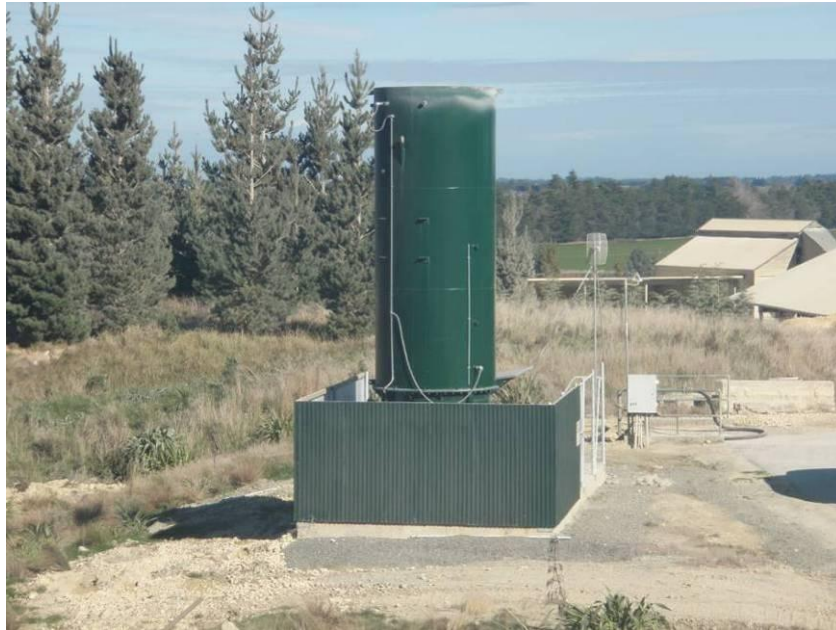
Figure 54: AB Lime permanent gas flare
