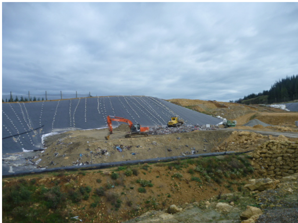
Figure 18 - Heavy machinery filling a new section of the AB Lime Limited landfill with waste. In the background is the liner used to cover sections that receive waste. In the foreground is the drain used to collect the stormwater.
