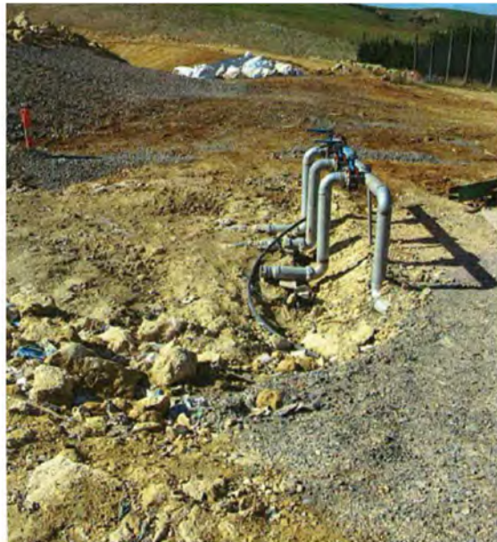
Leachate reticulation pipework and valves
