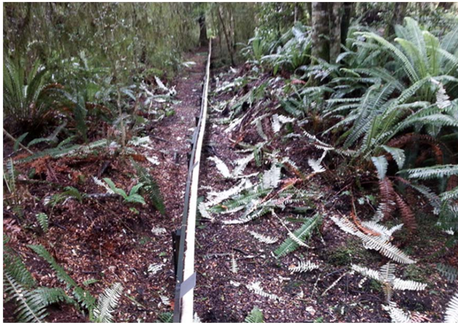
Moturau Hut discharge pipes.
