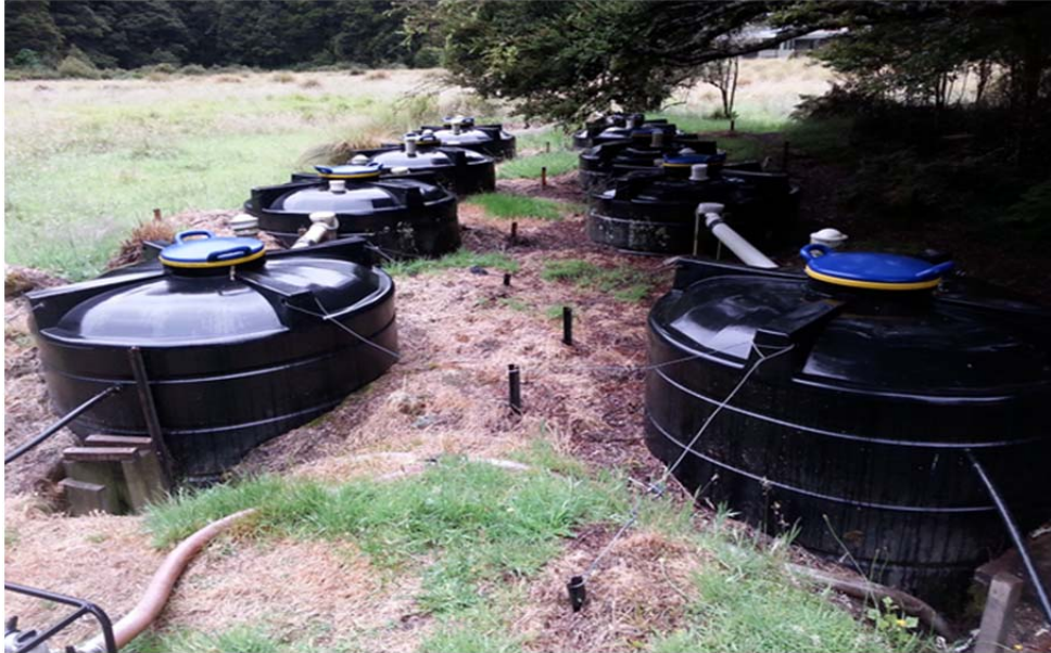
Iris Burn Hut discharge holding tanks.
