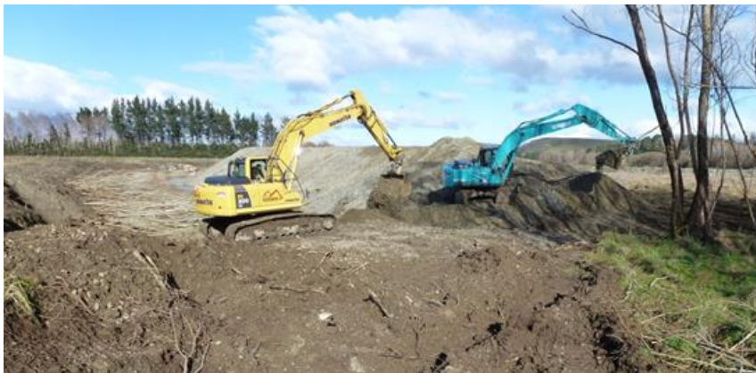
Clearing/replanting of willows and gravel extraction on the Whitestone River in Te Anau.
