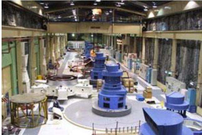
Manapouri Power Station.
