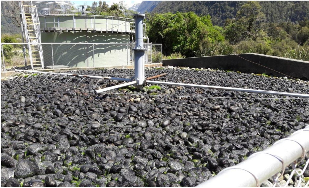
Milford Sound Wastewater Treatment Plant
