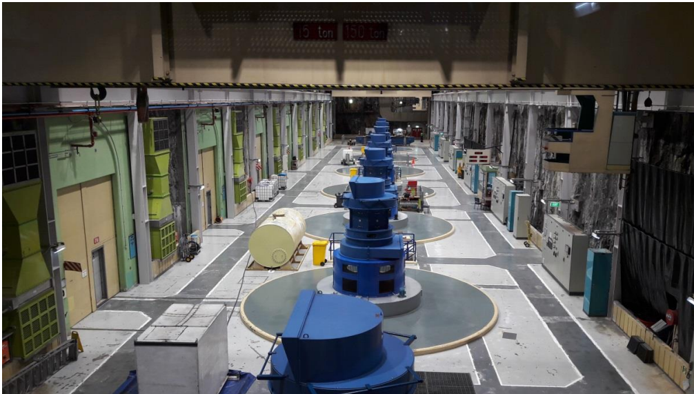
Manapouri Power Scheme
