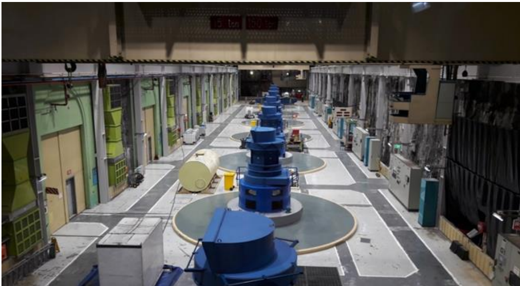
Figure 10: Turbine Hall - Manapouri Power Station
