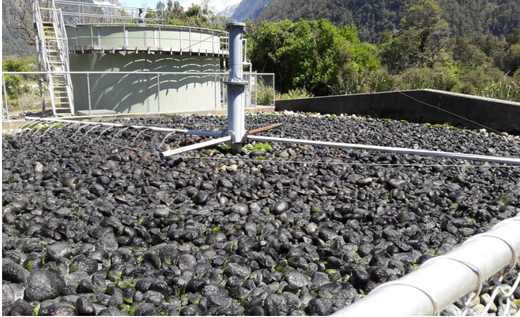
Figure 20: Milford Sound wastewater treatment plant
