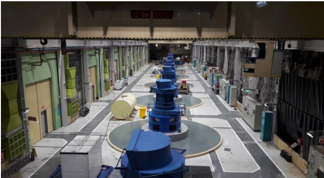
Figure 12: Turbine Hall - Manapouri Power Station
