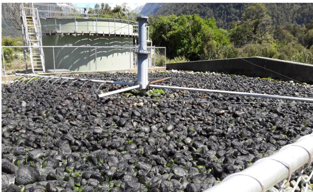
Figure 22: Milford Sound wastewater treatment plant
