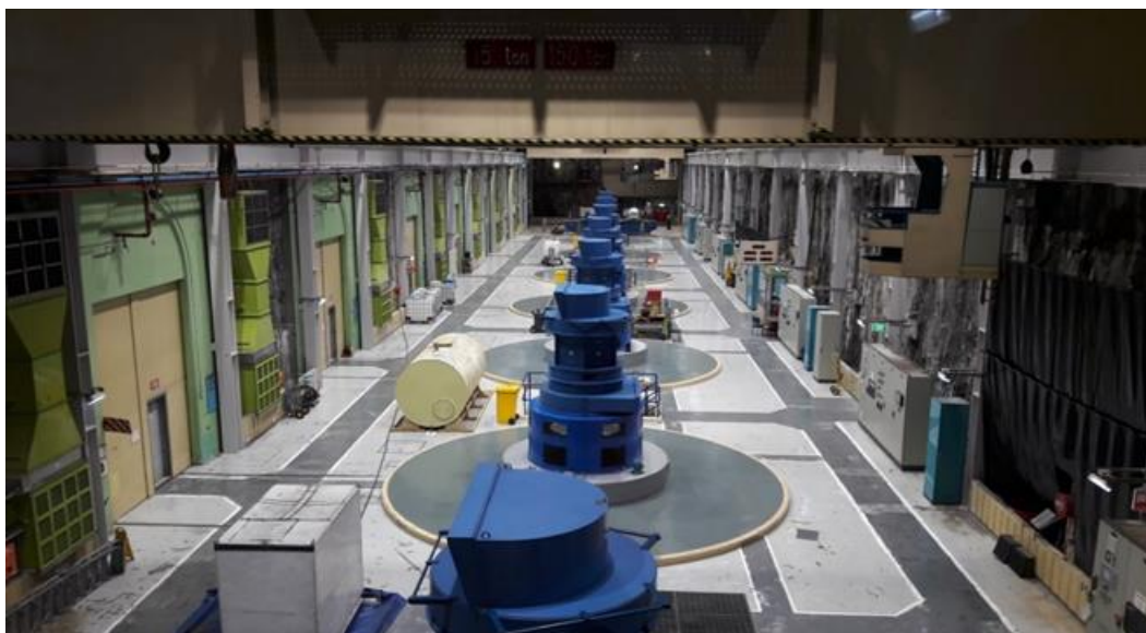
Figure 10: Turbine Hall - Manapouri Power Station
