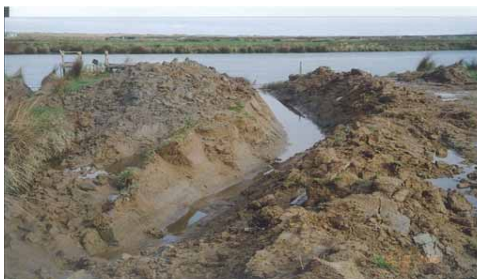
Figure 55 - Unauthorised excavation on Mataura River
