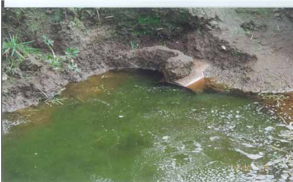
Figure 44 - DSE flowing from clay drainage tile
