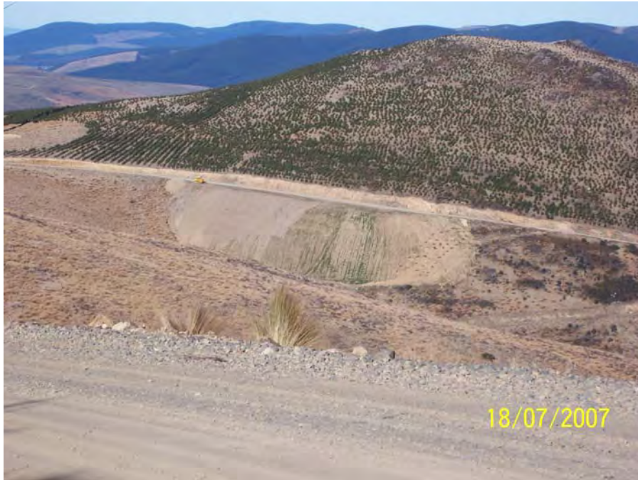
Figure 40 -A view of an area adjacent to the roadway that has been hydro-seeded
