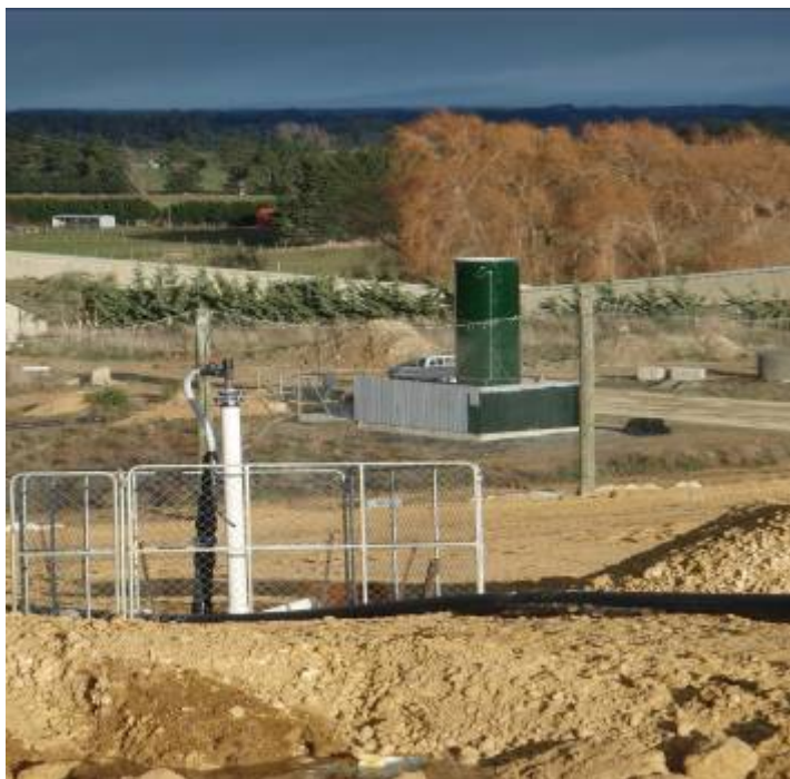
Figure 61 - Gas extraction well (front left of picture) and permanent flare (rear green structure)
