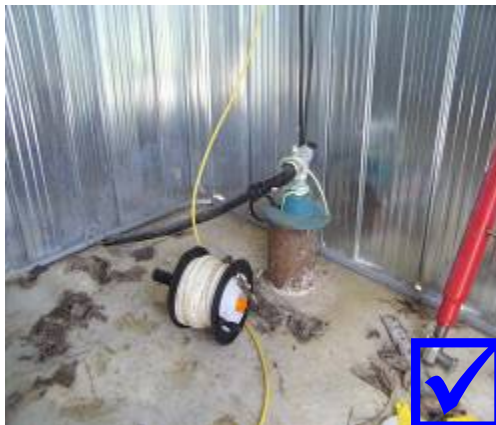
Figure 27 - Excellent bore construction and protection
