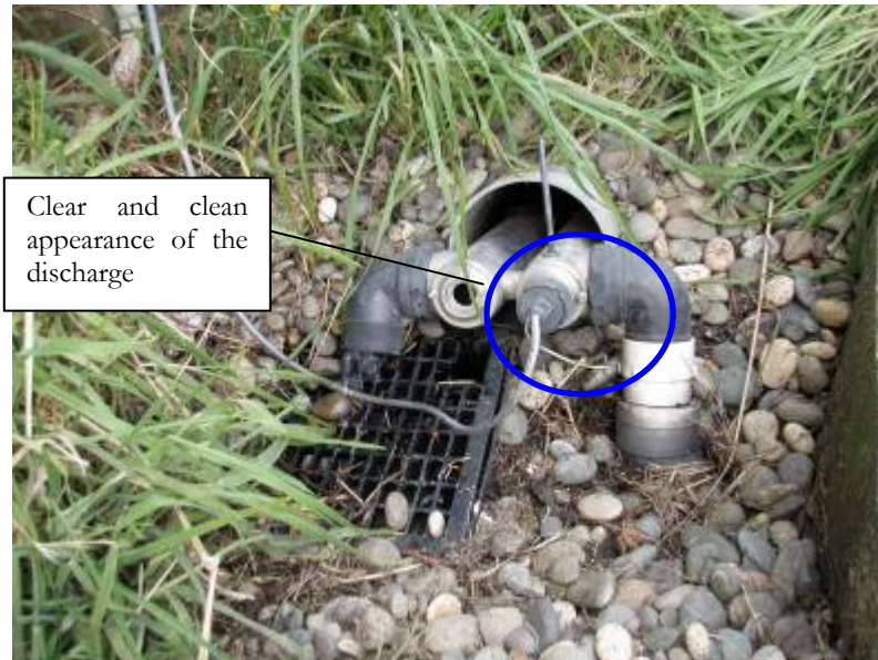
Figure 49 - Sewage treatment system discharge after final UV treatment
