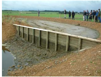
Figure 8 – Weeping wall solids separation
