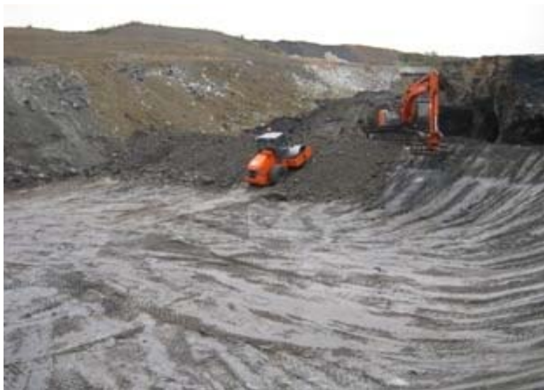
Figure 63 - Diggers forming cell lining for relocation of Nightcaps landfill – photograph supplied by Takitimu Coal Limited
