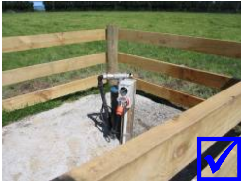
Figure 25 - Excellent bore construction and protection
