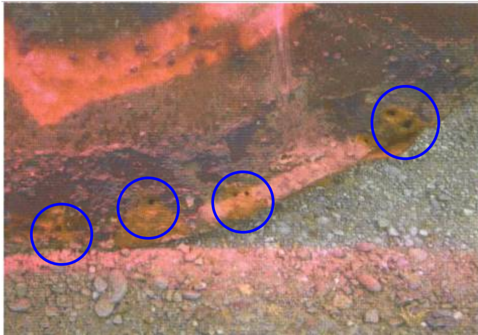
Figure 4 - The areas within the blue circles indicate holes found in an underground storage tank once it has been removed
