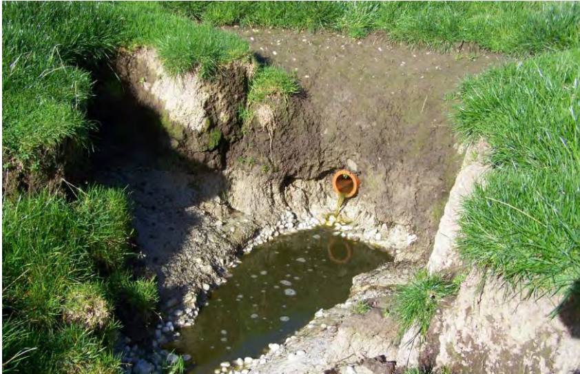
Figure 35 - Discharge of dairy shed effluent to a waterway from a tile drain.
