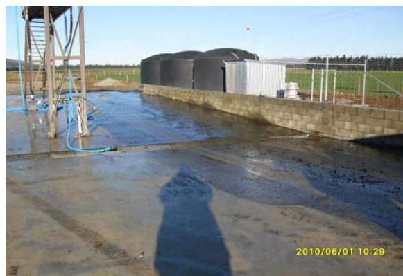
Figure 19 – Containment facility – washwater.
