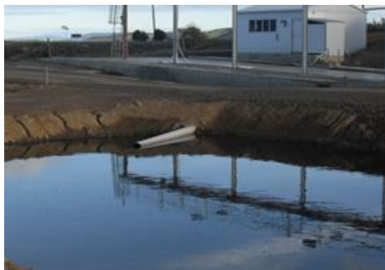
Figure 10 - Truck wash layout viewed from the settling pond, looking back at the cleaning pad.
