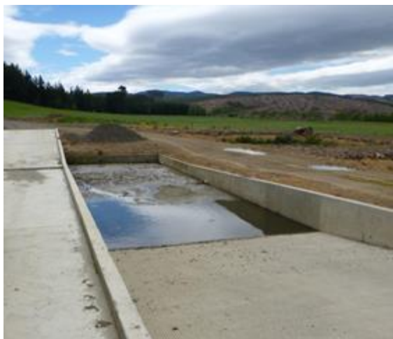
Figure 9 - Wash water from the cleaning pad (left) flows to a stone trap (centre) to collect the larger solids then out to the settling pond (far right).
