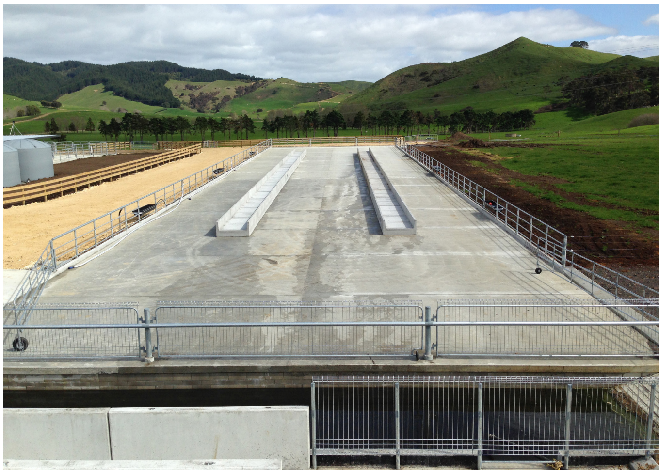
Typical stockholding area (feed pad) example that has an impermeable base. If your stockholding area does not meet the minimum permeability standard you will need to apply for resource consent. Note that you may need a consent or variation to your current consents for effluent storage if you have an impermeable stockholding area. (Photo: Don Chapman – Chapman Dairy Ltd)
