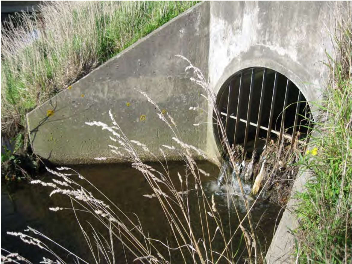
Figure 9 View of a stormwater drain entering Otepuni Creek (left) near Lindisfarne Street, Invercargill. View taken from true left, April 2016.
