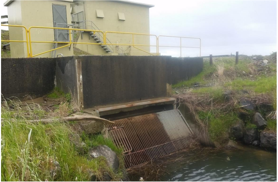
Figure 12: View of the Alliance water take structure.
