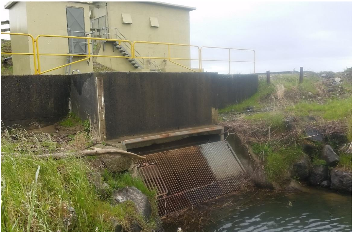
Figure 6: View of the Alliance water take structure.
