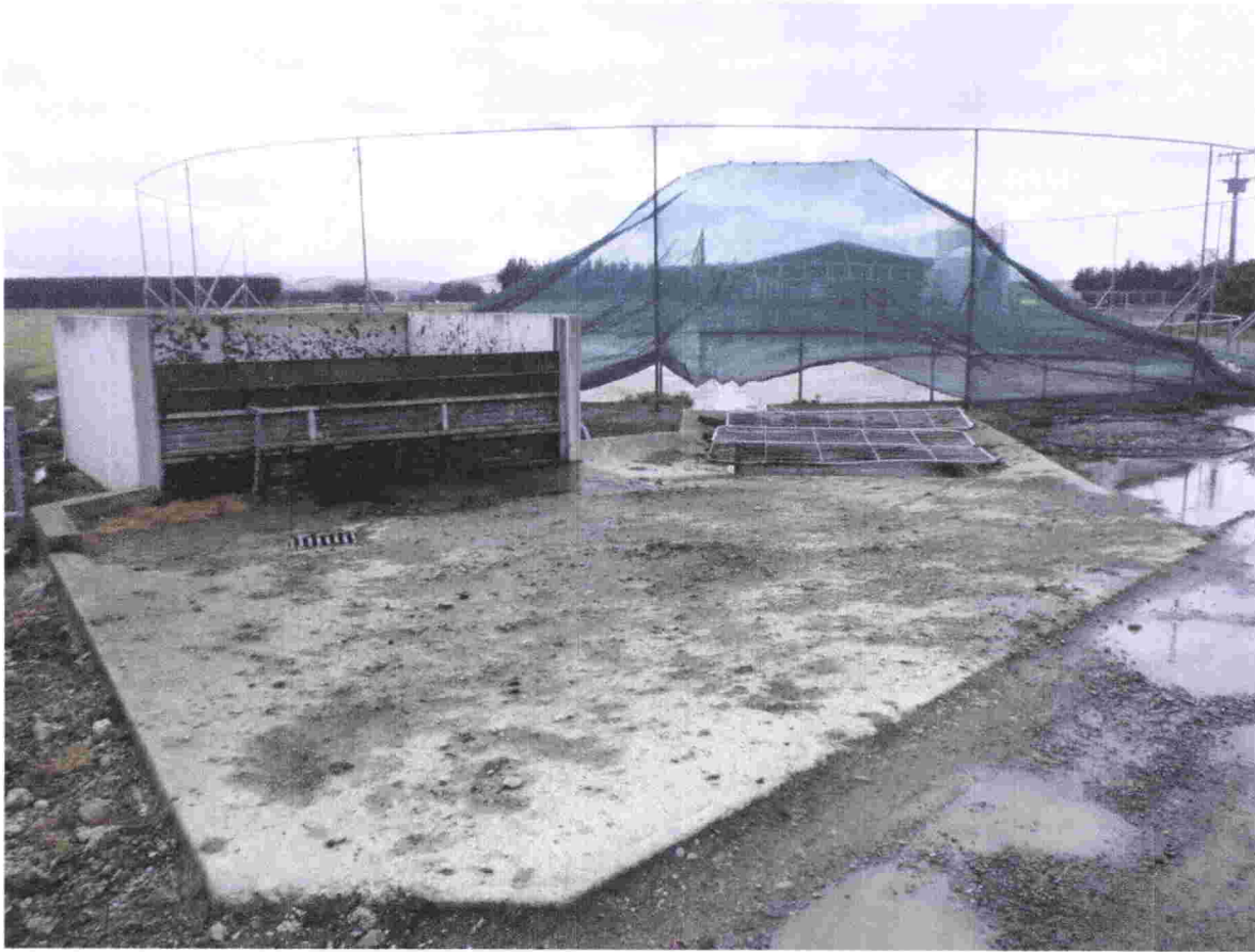
Stone trap – right and sludge bunker with weeping wall
