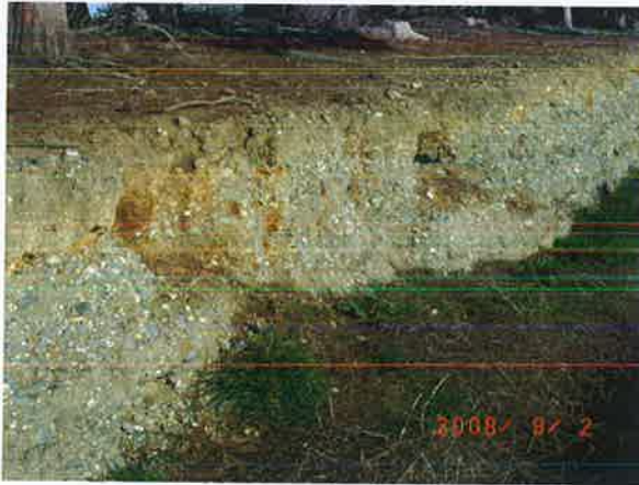
▪ Figure 4: Photograph of the construction of the Charlton saleyard settling pond walls (2 nd September 2008)
