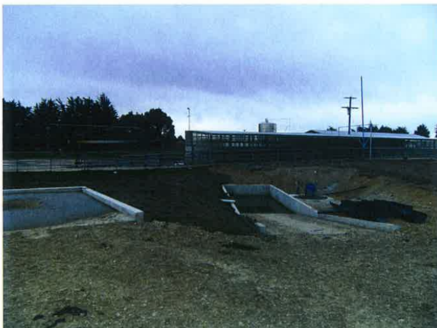
Figure 7. Upgraded sump and solids pad.
