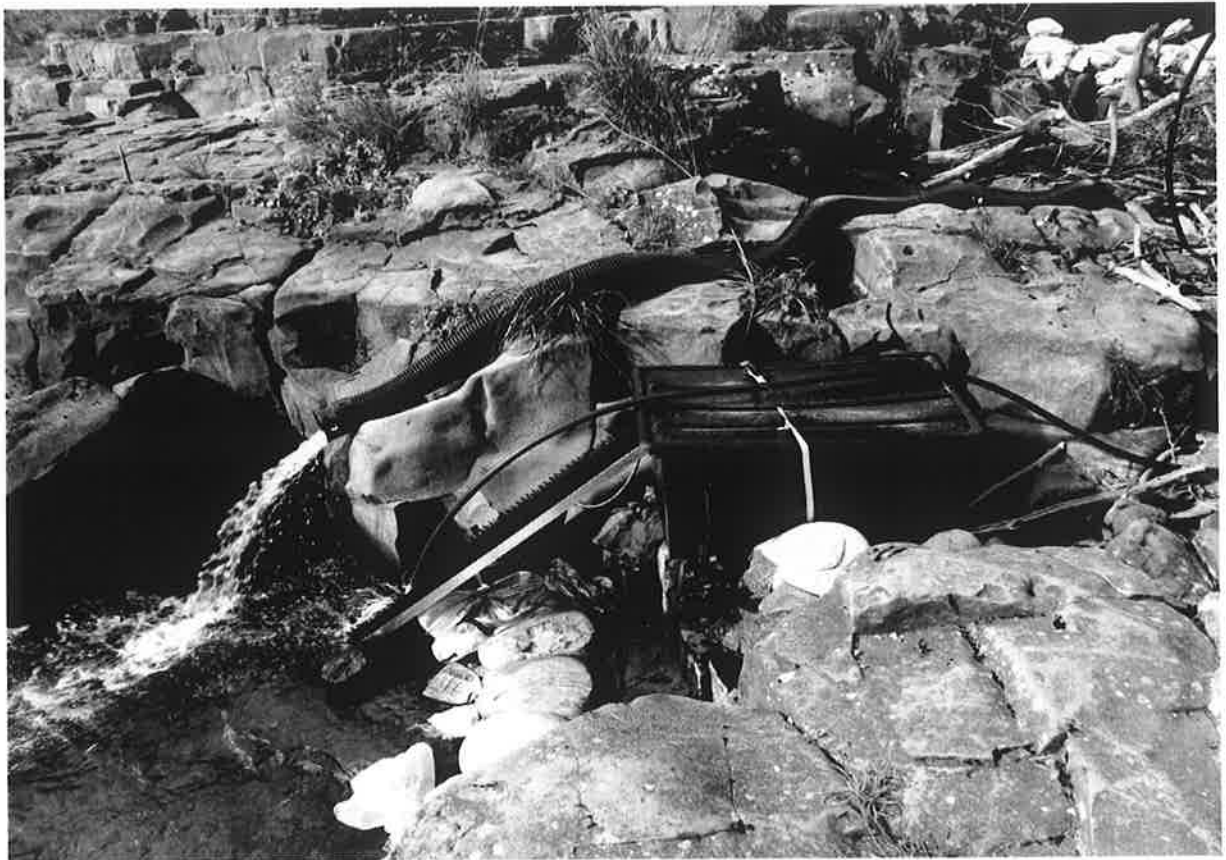
Fig 1. The trap in situ. The corrugated pipe discharges leakage water from the sluice gate which would otherwise travel over the rock channel where the trap is sited. The sticks to the right are the dumped trash rack debris.
