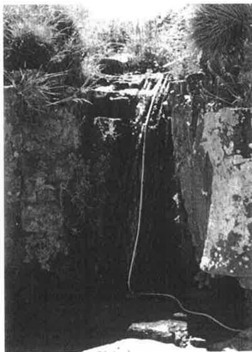
Figure 2-2: Close-up photo of the cap rock with possible passage opportunities/provision for elvers. Spat ropes to facilitate upstream passage of elvers and other fish have been installed at this location. (From HES 2016a.)
