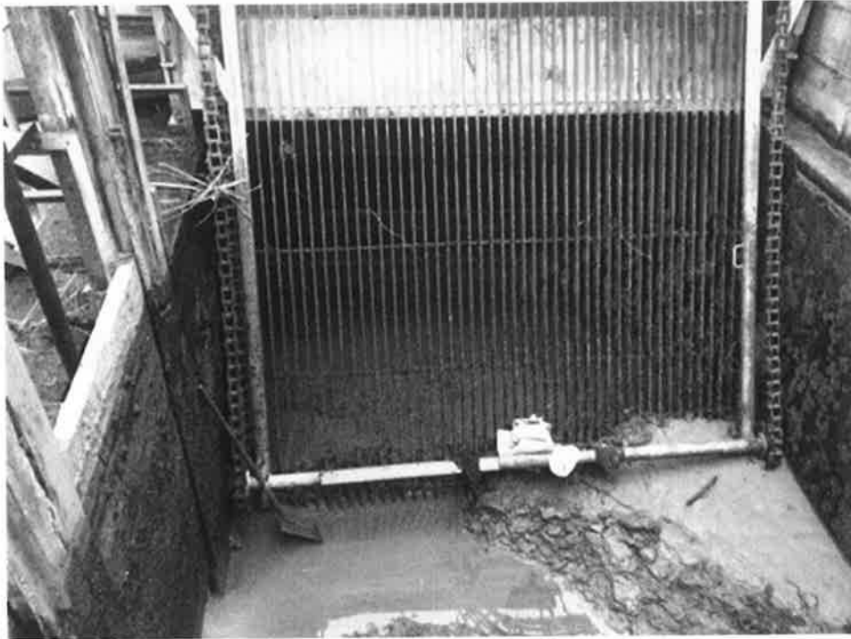
Figure 3-5: Dewatered trash screen. Note silt deposit at bottom of intake. This may indicate reduced velocities which could be used by eels to avoid impingement and entrainment. Photo courtesy Alliance.
