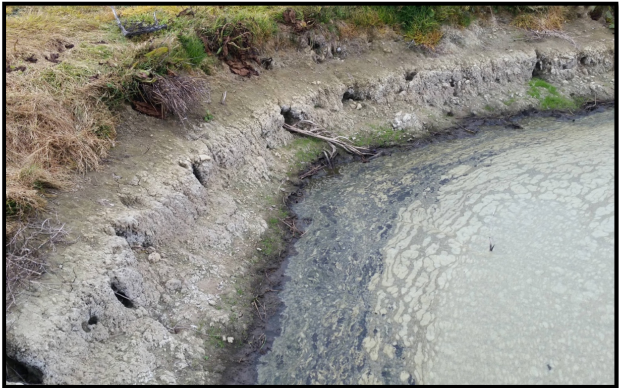
Figure 1: Holes in the internal embankment of the pond
