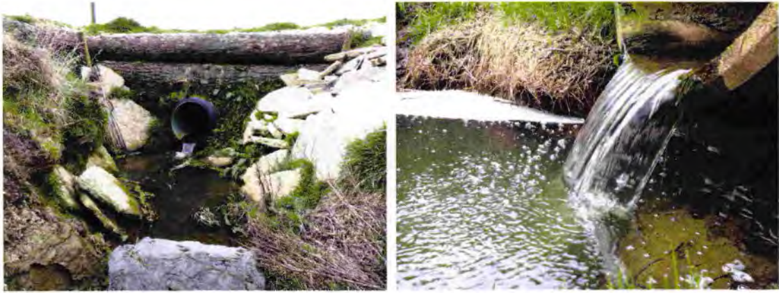
Figure 8 Two culverts in Waituna Creek tributary at Amtink Farm where fish passage should be improved, October 2016.
