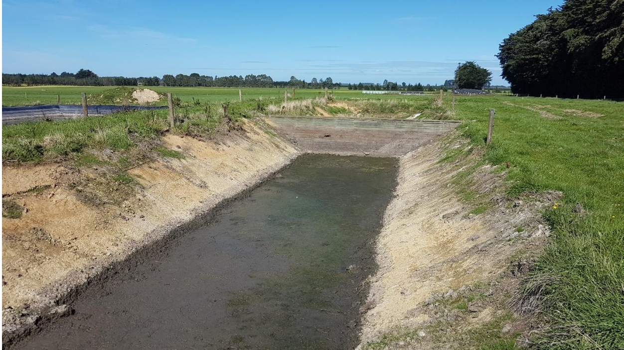
Figure 4: Double sludge bed with weeping wall
