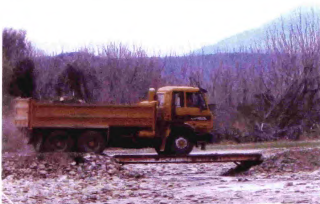
Photo 14 – Looking South and Downstream Shows Temporary Access Bridge Positioned Across Active/Inactive Runner Separating Areas A1 & B
