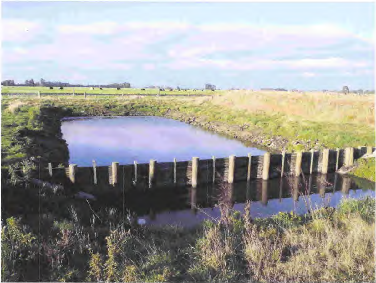
Weeping wall in sludge bed
