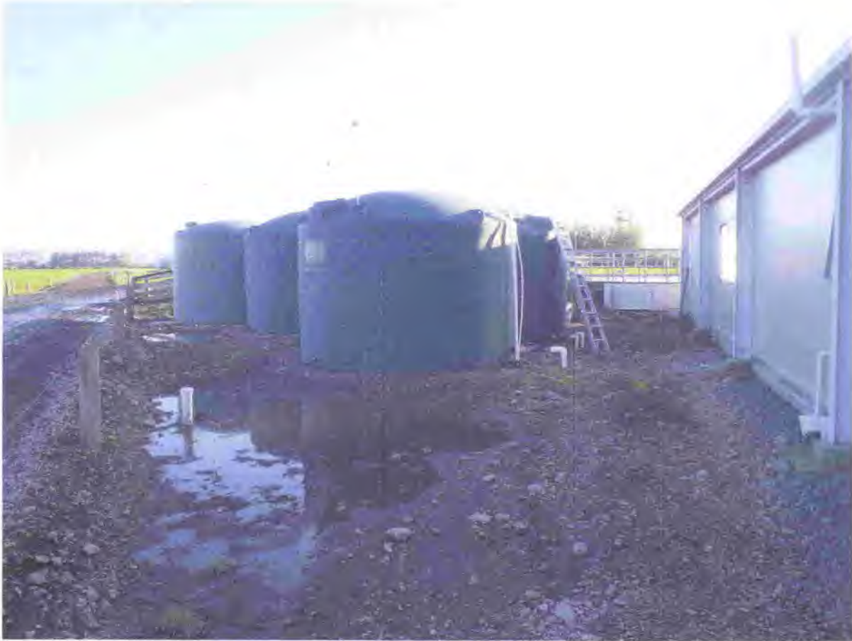
Water storage tanks
