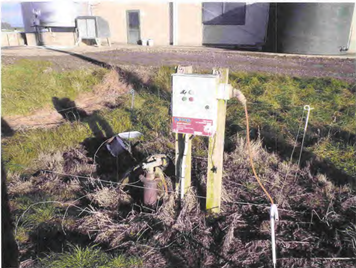
Bore in tanker track
