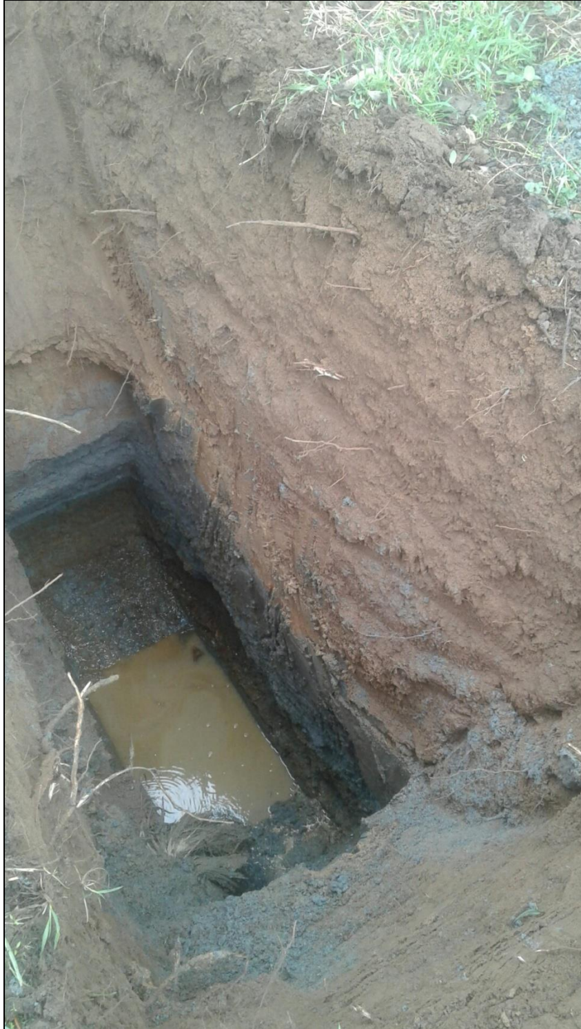
Figure 1. Subsurface geology exposed in a test pit adjacent to the Tokanui WWTP site.
