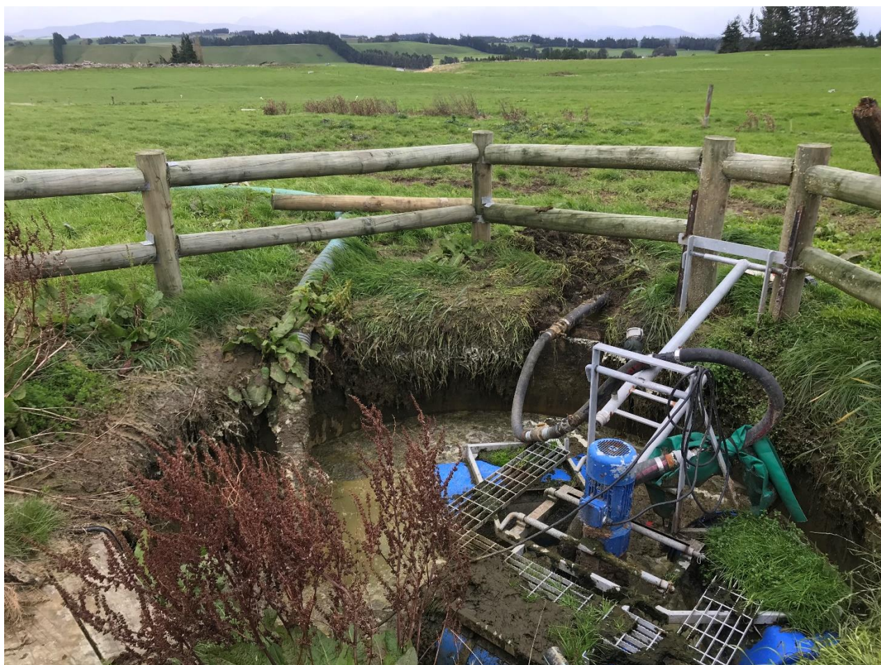
Figure 2: The pump sump near the dairy shed. This has been included in the revised Massey Pond Calculator as additional effluent storage.
